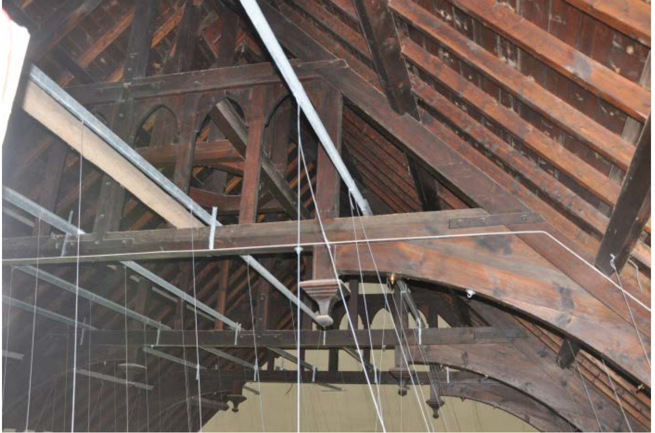
Roof space hidden above the suspended ceiling you see in the next picture.
